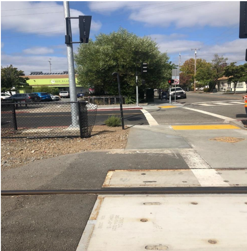
5 th Street, San Rafael- Flat work completed and Fence installation in progress
