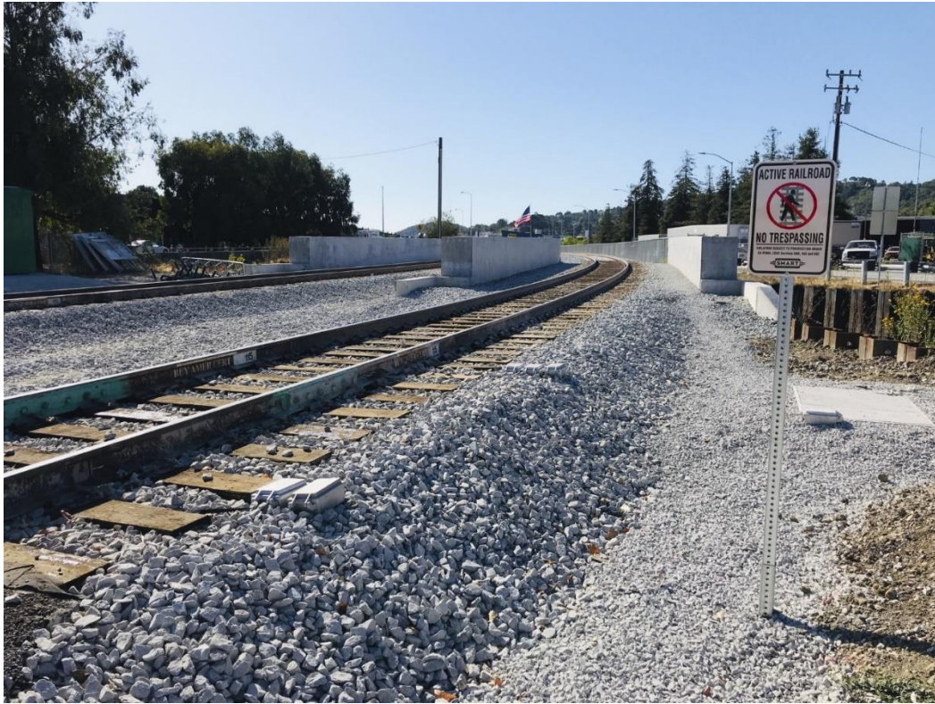
2 nd Street crossing – NO Trespassing Signs Installed
