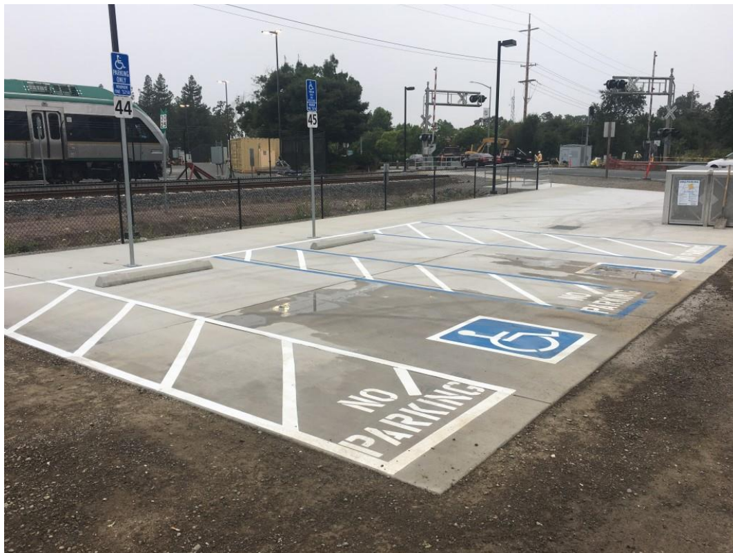
The completed concrete pad for Handicap Parking and Electric Bike Locker at Airport Station
