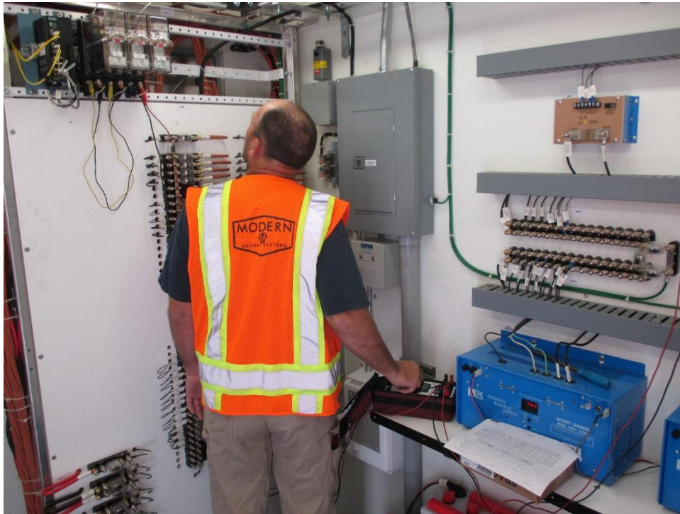
Contractor Technician performing traffic signal interface testing, North Santa Rosa
