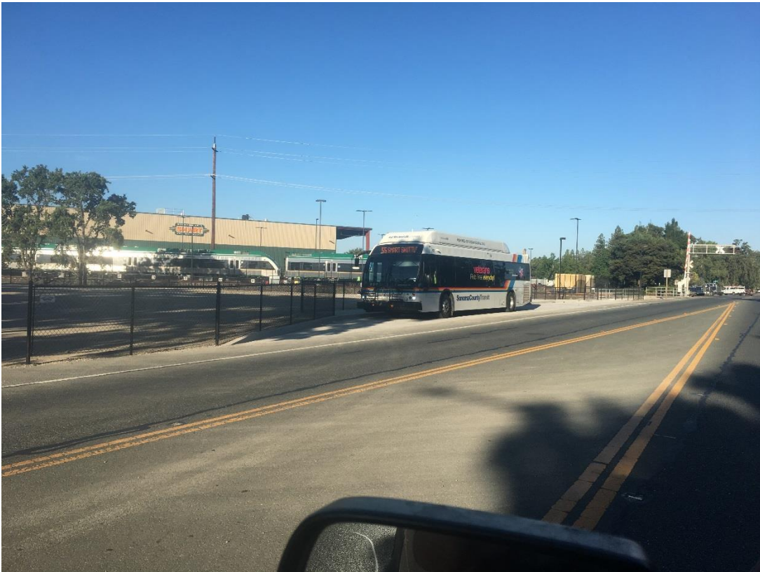
Joint Project with Sonoma County - New bus pull-out and sidewalk at the Airport Station parking lot
