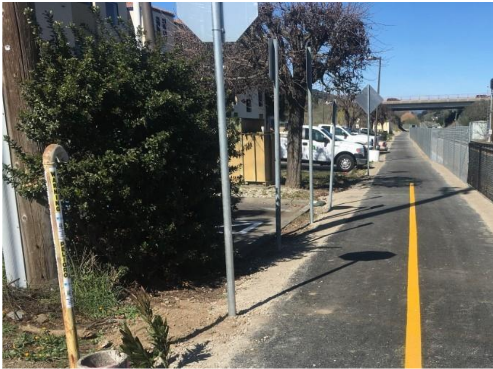
Pathway from Novato San Marin station to Rush Creek Place is complete.
