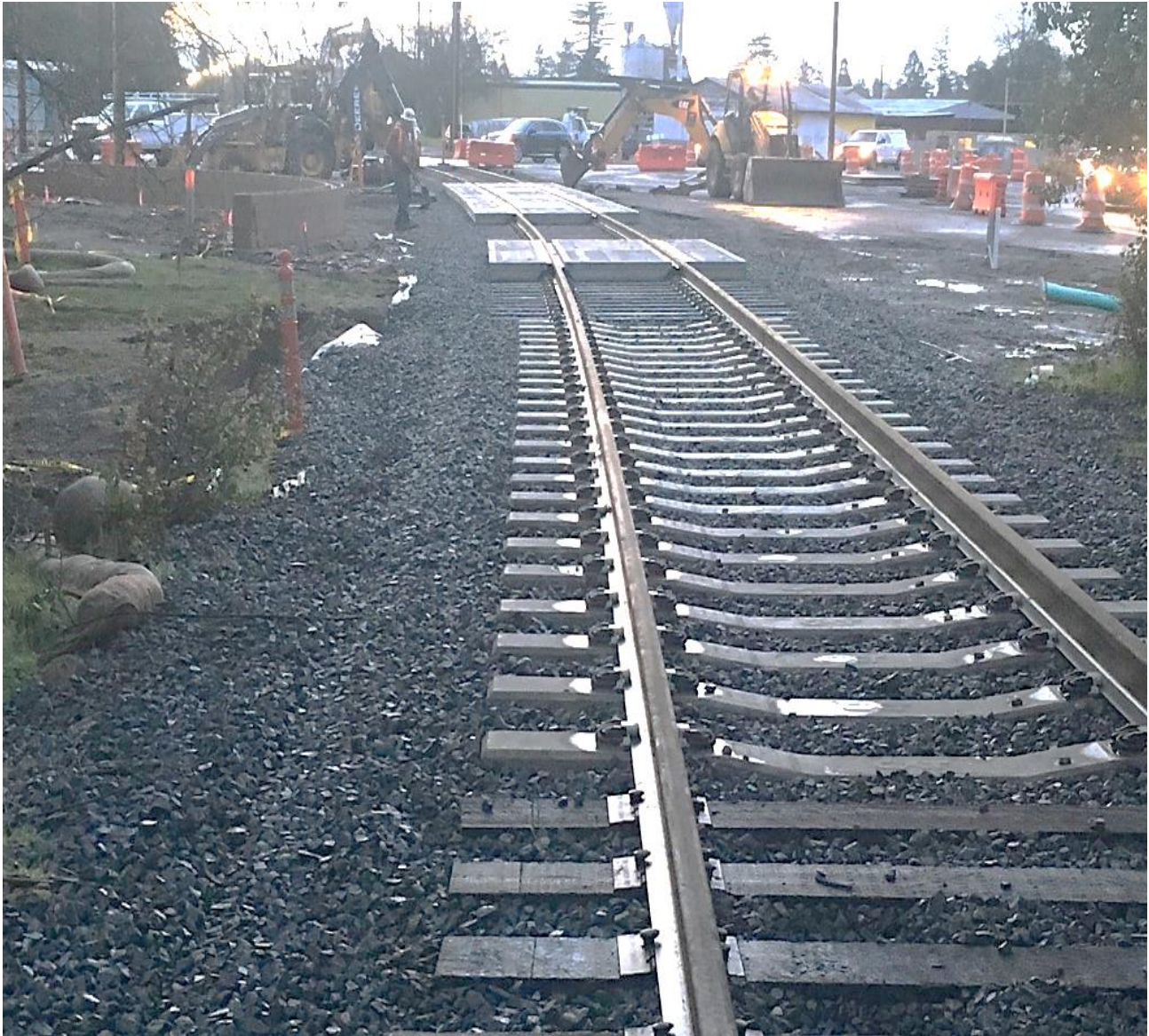
Track only reconstruction through the Healdsburg 5-way roundabout consisting of new ballast, ties, rail, and crossing panels was completed March 14, 2018
