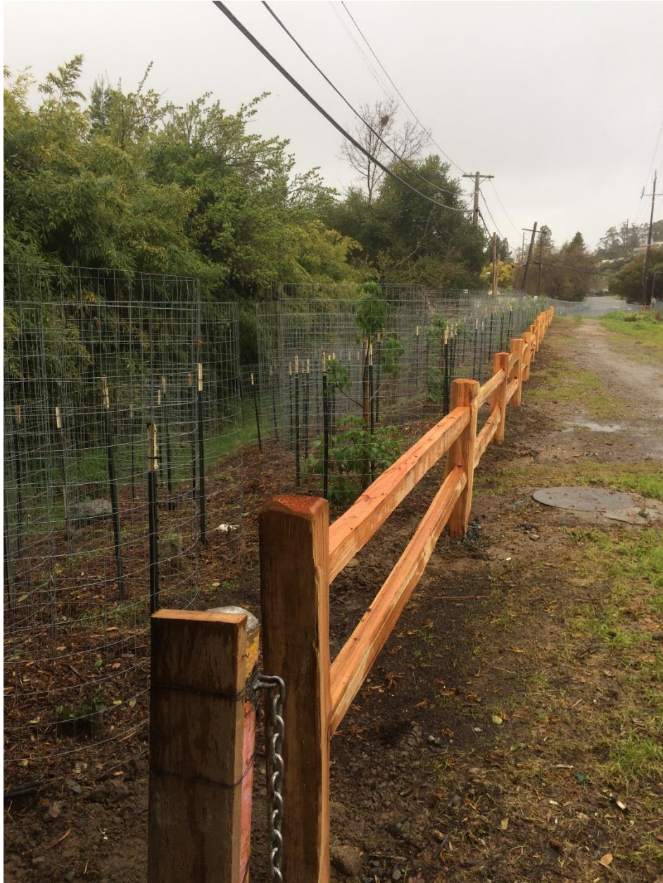
Completed riparian mitigation near the Civic Center Station to offset impacts from the pathway construction
